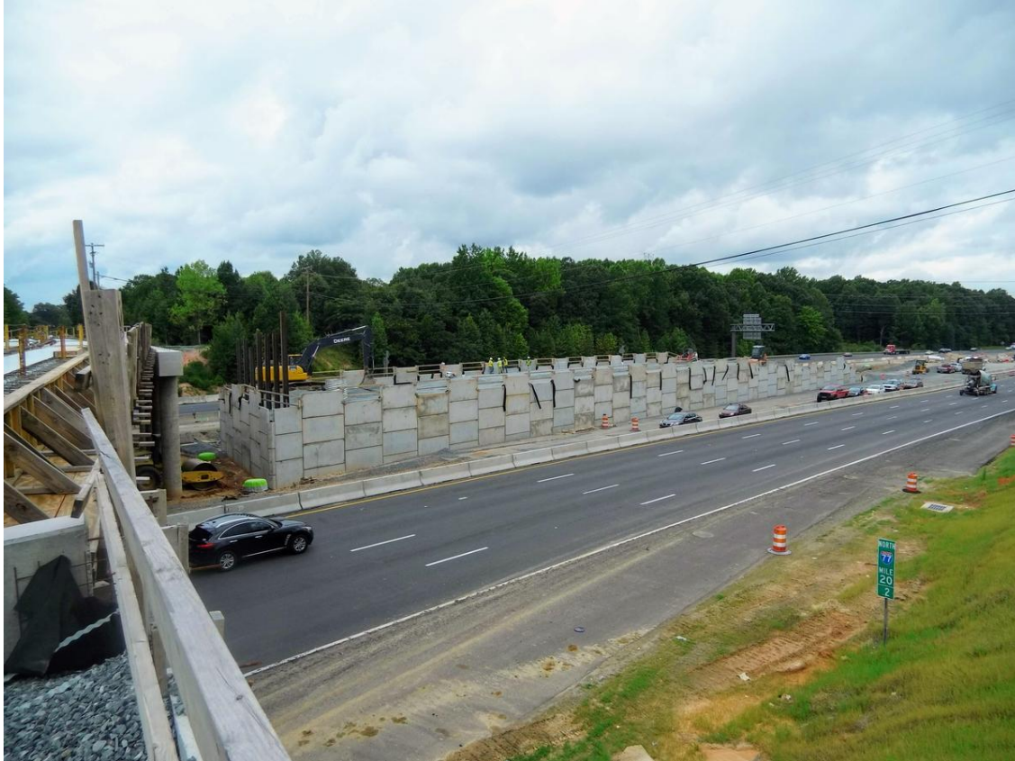
A direct access ramp is being added at I-77 and Hambright Road in Huntersville. Officials say it won't be open until after the toll lanes open. CREDIT DAVID BORAKS / WFAE
