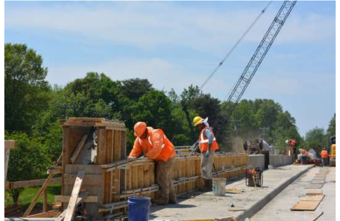
Building sidewalks and hand rails at the new Griffith Street bridge in Davidson.
