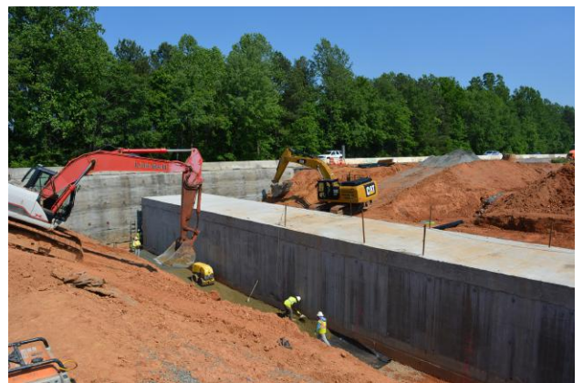
Backfilling activities at the Torrence Creek pedestrian culvert just north of Exit 23 in Huntersville
