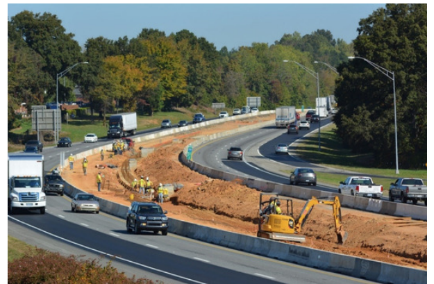
Crews working on the footing of the new permanent concrete safety barrier just north of Exit 28 (Catawba Ave.)
